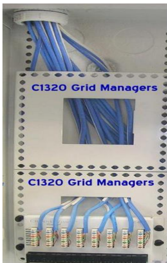
Fig. 7. Multiple CAT-5 cables from distribution point.
